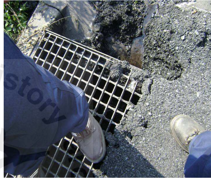
T1-06: Drain blocked with coal at the coal storage area
